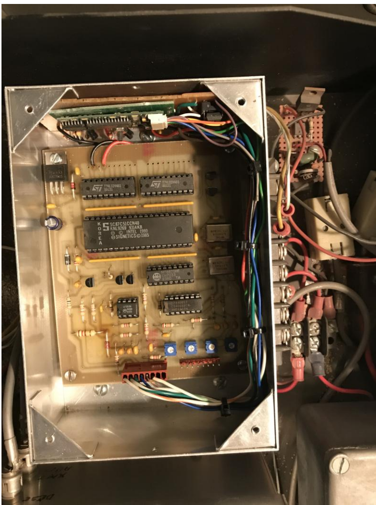
220 MHz repeater controller
