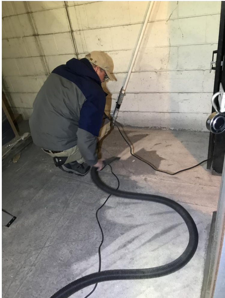
Dale, KB9JJA, doing some housekeeping around the repeater cabinets KC9MZ photo
